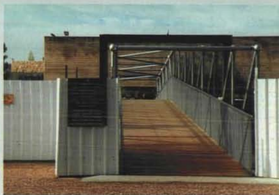
In order to accommodate visitors during the construction at Yad Vashem, two temporary foot bridges and a vehicle bridge, spanning the construction site have been erected and an outdoor lift for the handicapped is being installed. Above left: vehicle bridge, right: foot bridge. Below: foot bridge
