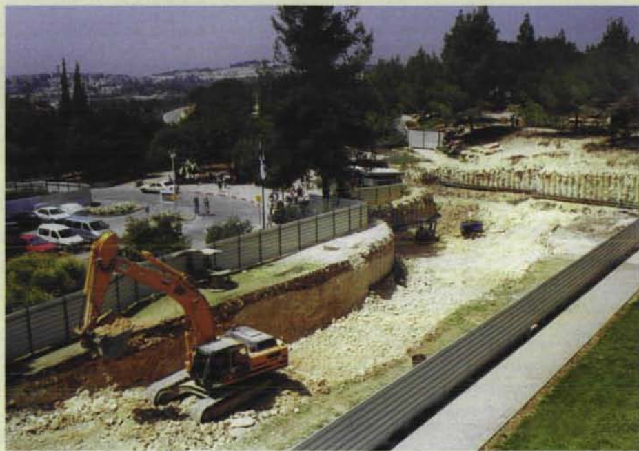
The construction of the Visitors Center (Mevoah) and parking facilities is progressing. The Visitors Center is being constructed with the generous support of David and Fela Shappell from Los Angeles, and with the assistance of the Government of Israel's Ministry of Tourism.
